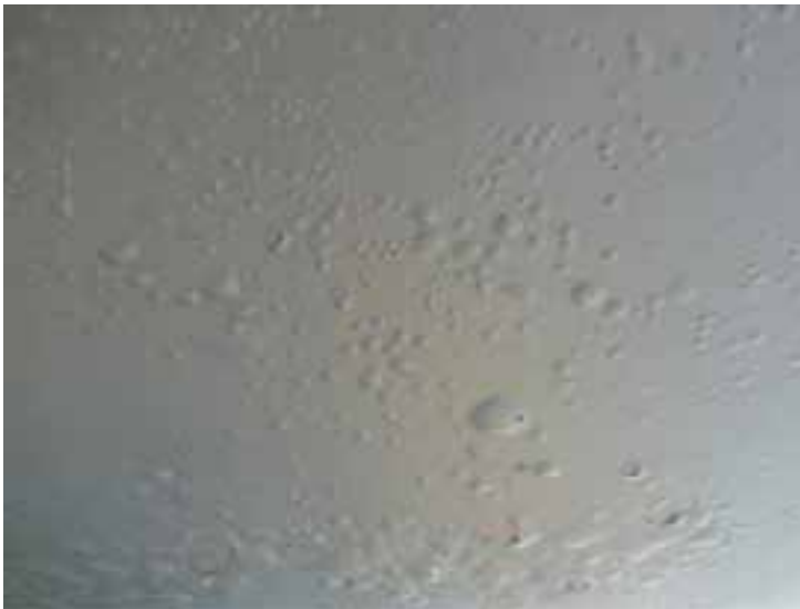
Osmoseschaden in fortgeschrittenem Stadium
